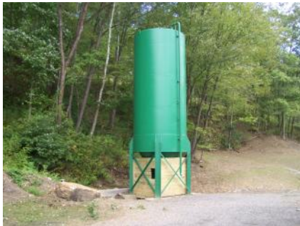
Lime dosing silo at Waterworks
